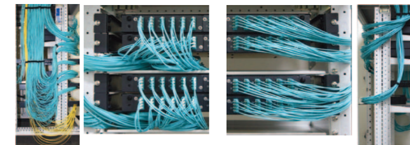
Conventional cabling solution
